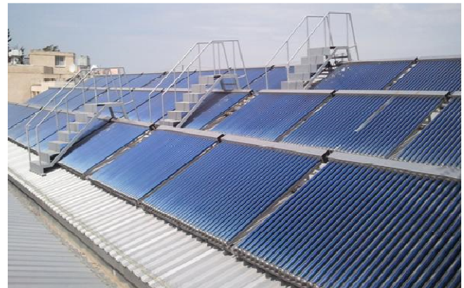
Fig. 3 Photo of one of the two banks of solar evacuated tube collectors
