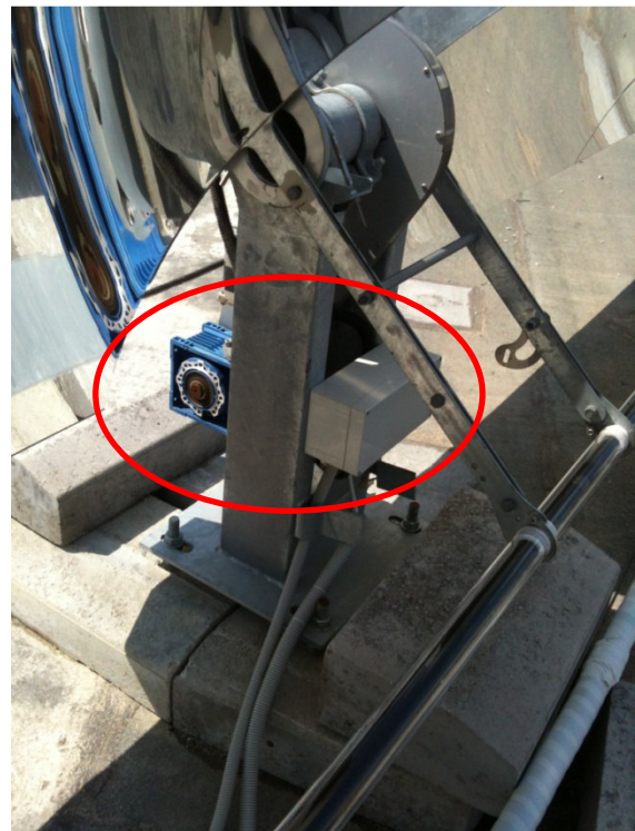
Fig. 2. Photo of the motor of the tracking system and central support of the collector (at park position).
